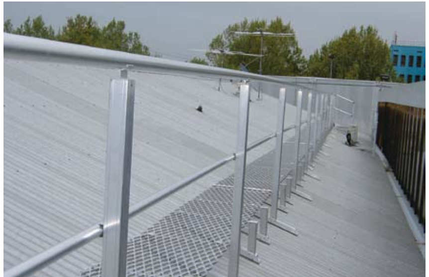
Walkways and guardrails are typical level 2 controls.
